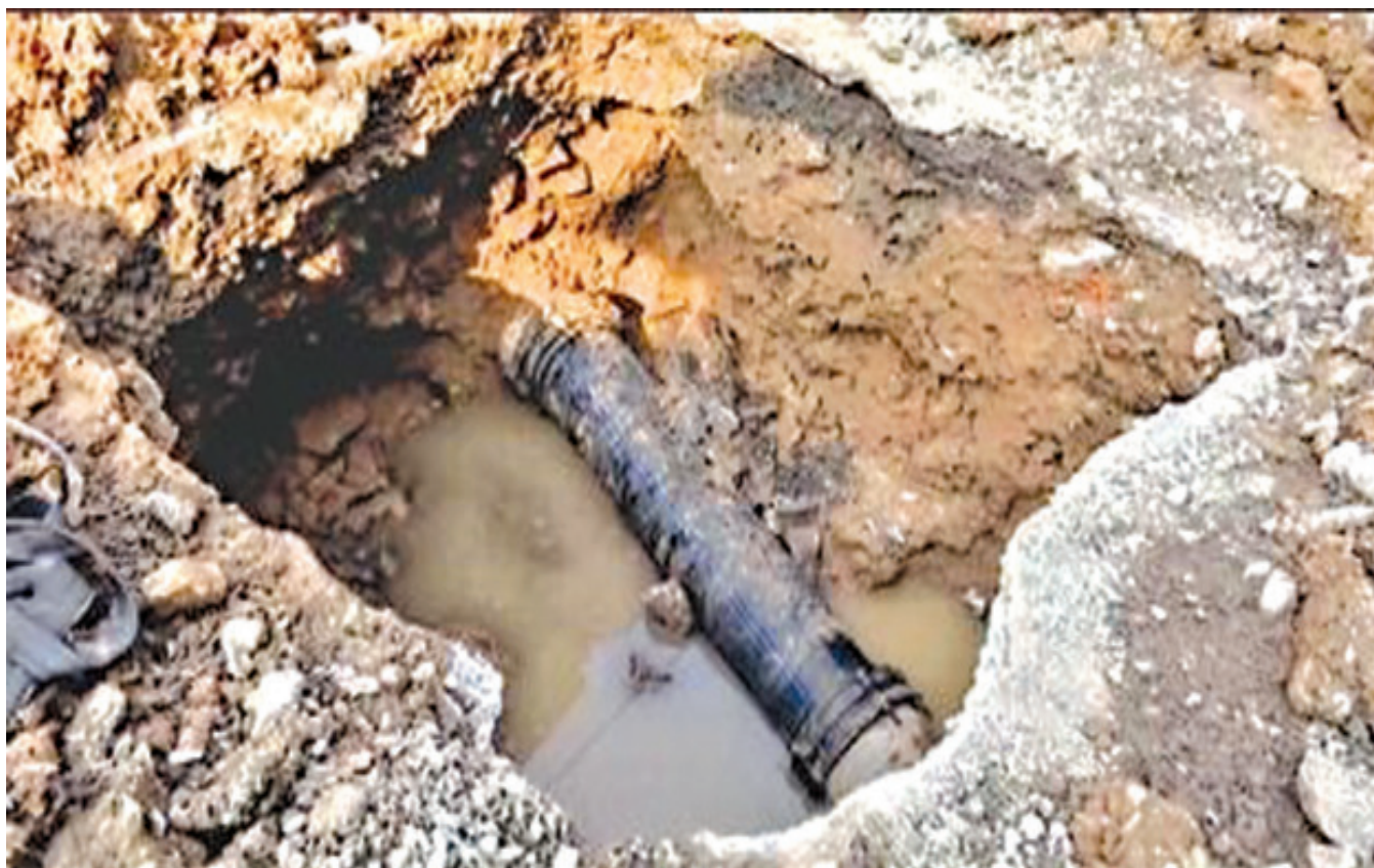
Figure 80: An exposed water pipeline in Indore's Bhagirathpura area.
