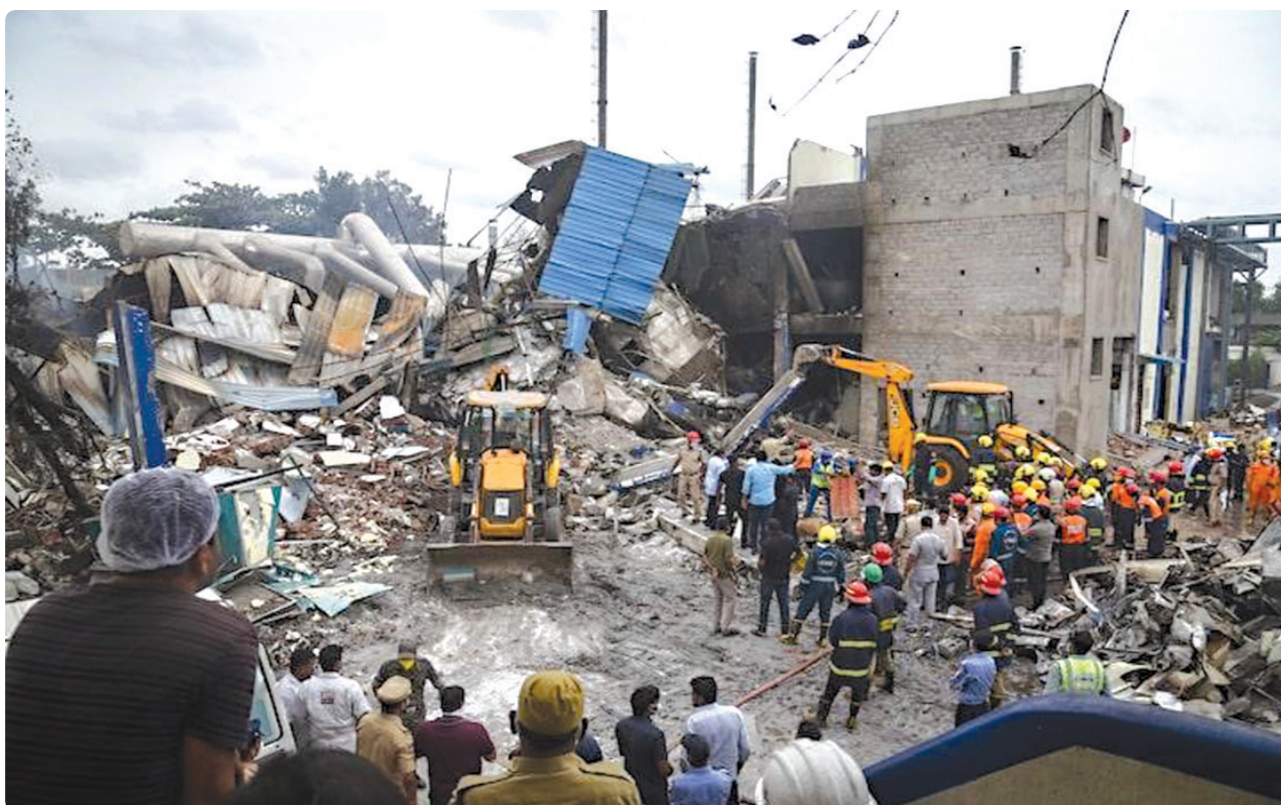
Figure 70: Rescue workers look for survivors after an explosion and fire at a chemical factory, in Sangareddy, in the southern state of Telangana, India, June 30, 2025.
